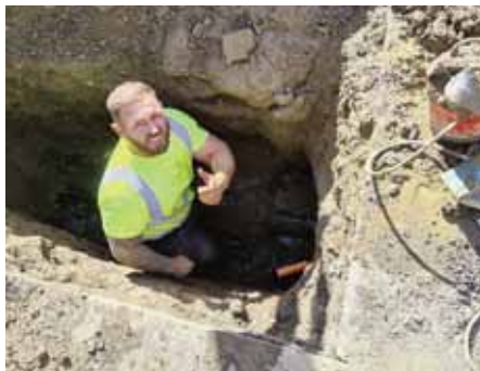
Thumbs up as another leaking water main is traced in Bradway
