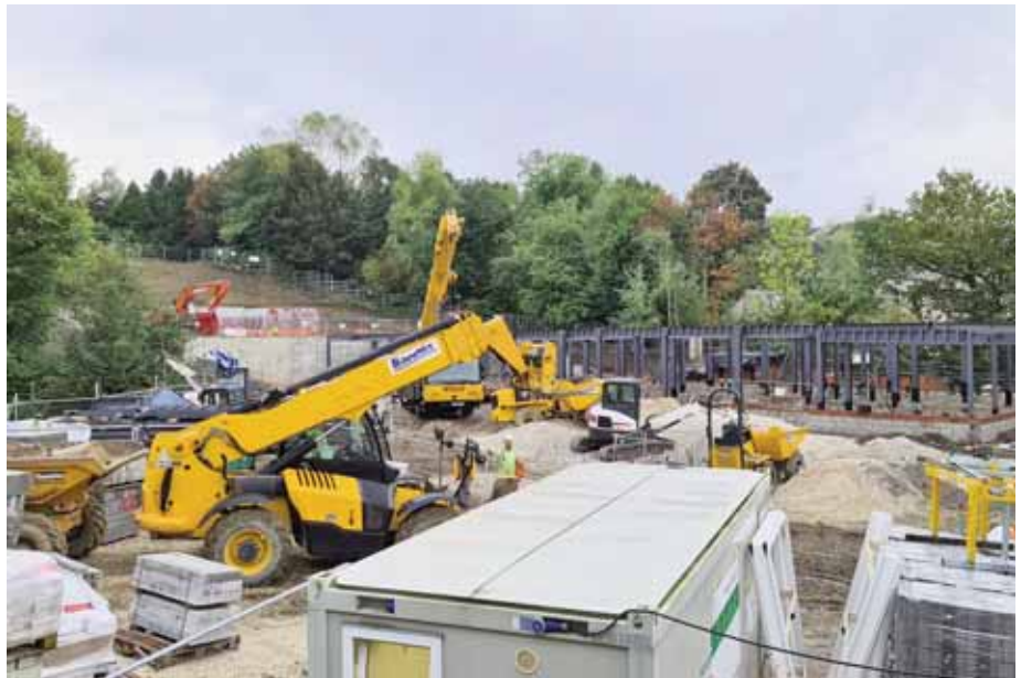
Building works at the new care home on Twentywell Lane. A very restricted site with little room to receive, store and then safely assemble all the various materials
