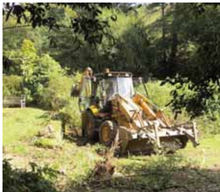
The Council moved in with a tractor and digger to clear all the overgrown shrubs.
