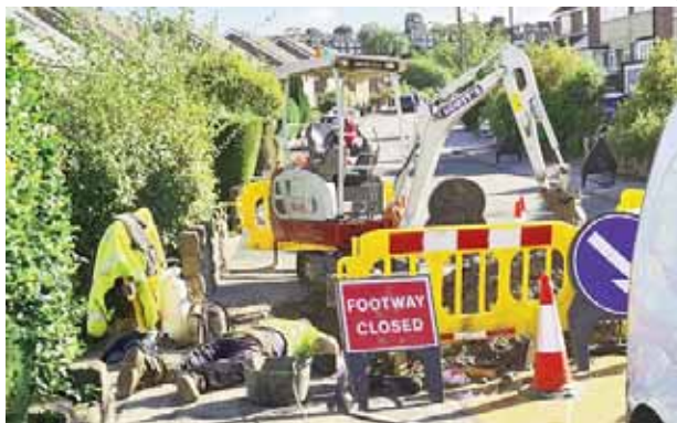
The familiar sight of footpath disruption in Bradway as the quest for leaking water mains continues
