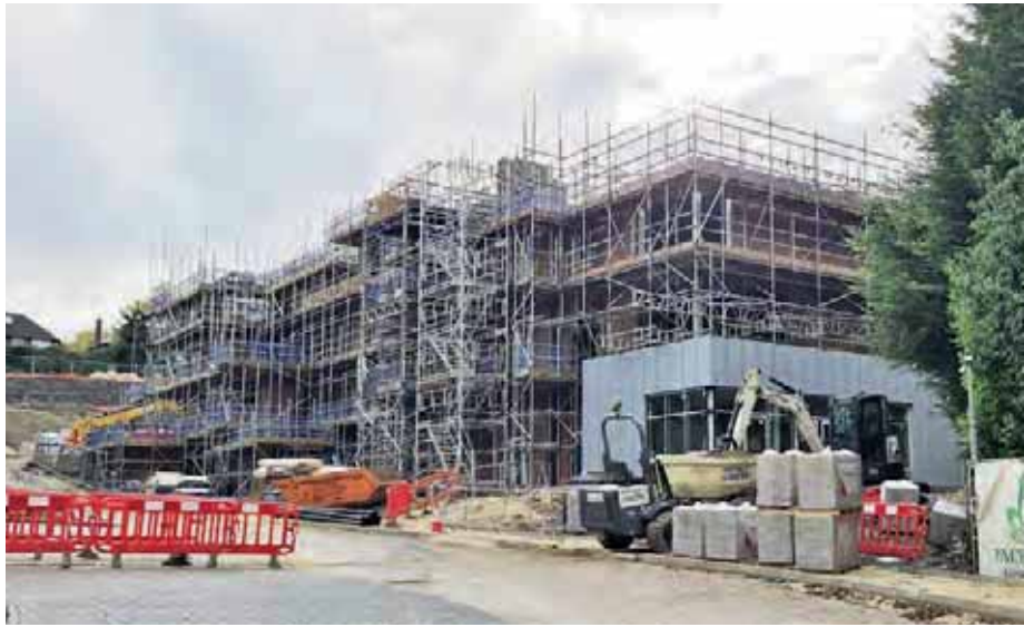
Outram Fields Care Home finally reaches its full height. Picture Chris Morgan
