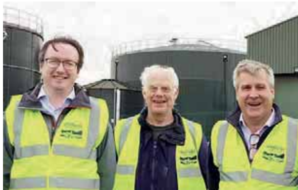
Joe Otten with cllrs Cliff Woodcraft and Tim Huggan on an inspection visit to the anaerobic digester
