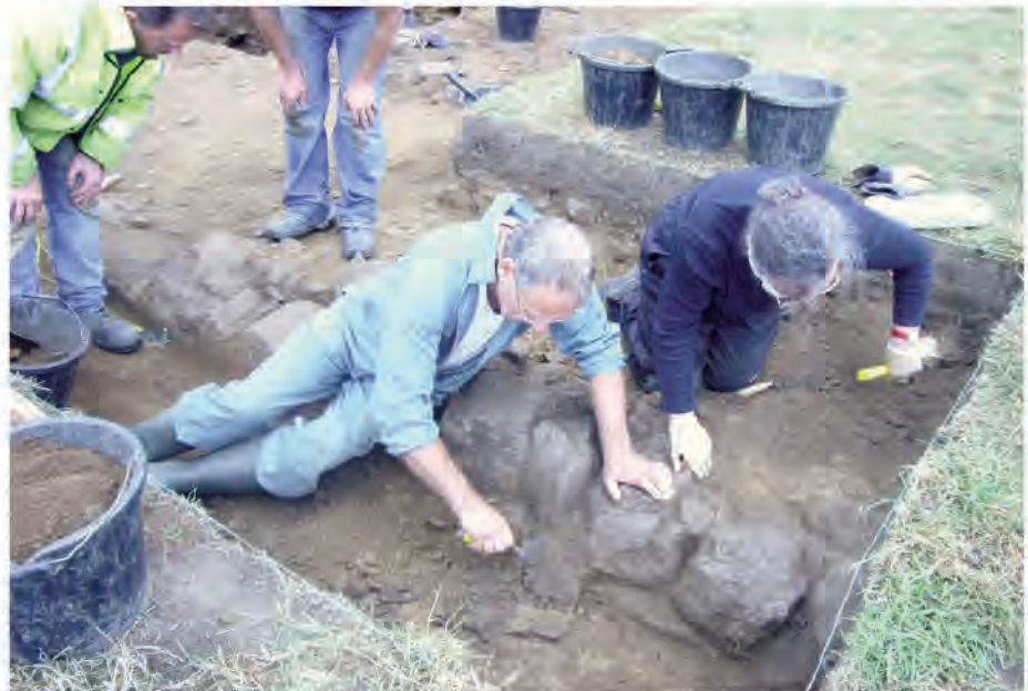
Members of The Time Travellers archaeology group excavating the foundations of a Roman building on Whirlow Hall Farm during 2011. It is believed that under the Roman building there are earlier Iron Age remains.
